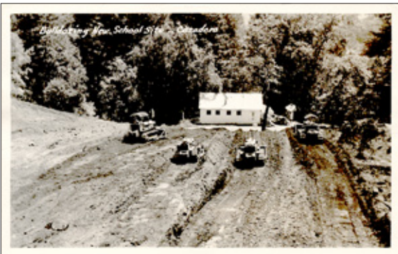
BULLDOZING : Local guys contributing skill and effort to building the new school, 1952.
